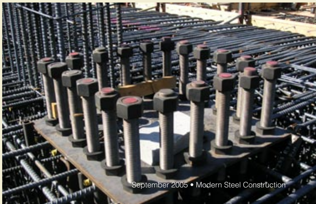
Below: Threaded anchor rods for a BRBF column prior to concrete placement. BRBF columns were taken through the reinforced concrete shear walls and connected directly to the foundation with up to 20 3"-diameter ASTM F1554 grade 105 anchor rods through base plates up to 9" thick. Photo courtesy Reaveley Engineers & Associates, Inc.
